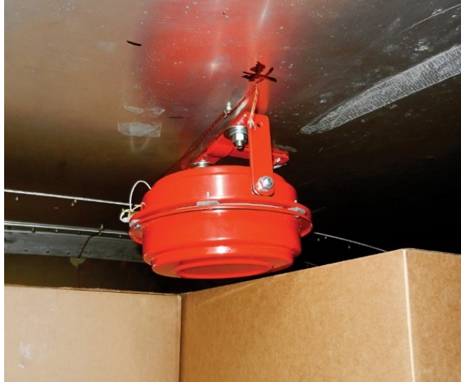
Figure 6.2 – In-container fire suppression system
